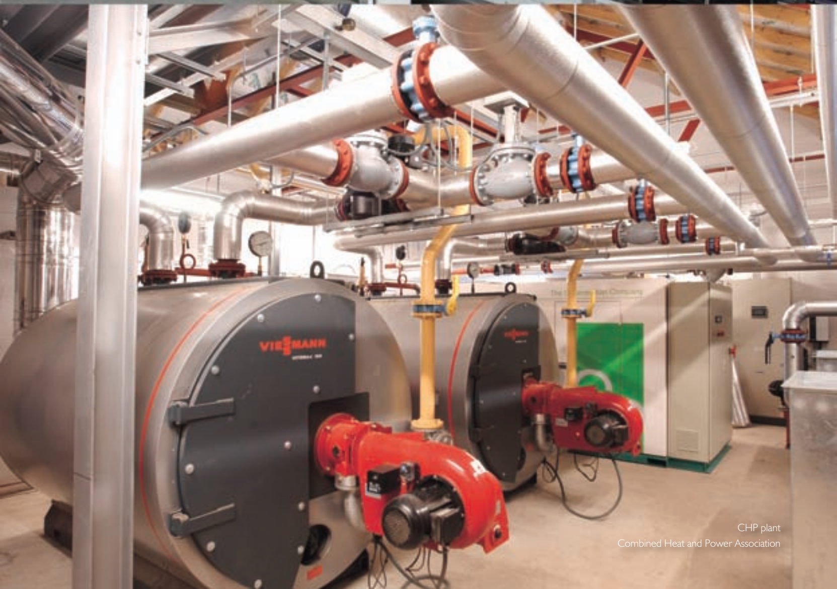
CHP plant E.ON
