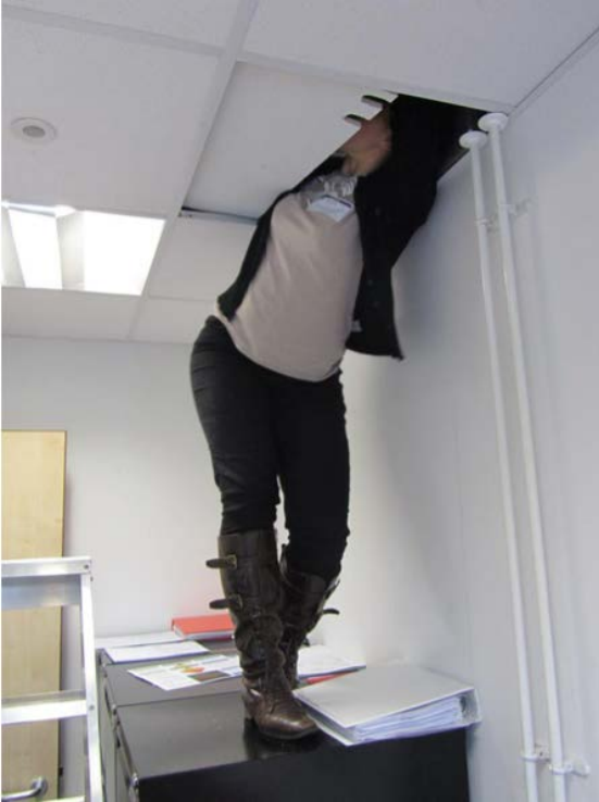
Poor placement of hot water meter
